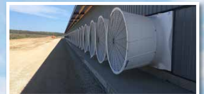
The cross ventilation system in the new barn not only keeps the cows more comfortable, it also increases the air quality flowing through the barns. Our goal is to have nearly equal air quality inside as outside on a year-round basis.
