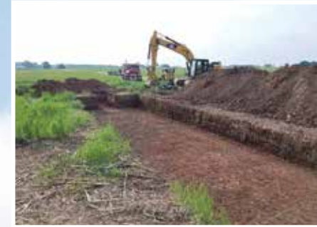
A five-foot deep trench is dug at the edge of a field.
