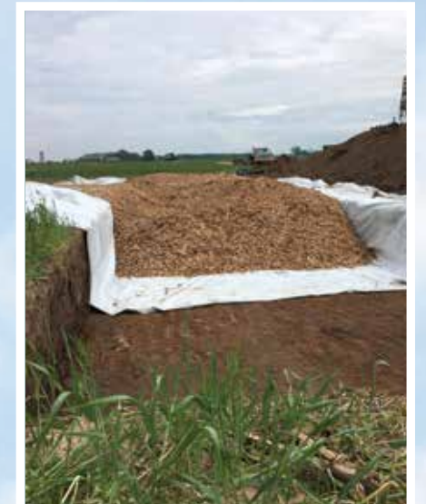
After a geotextile or plastic lining is installed, the trench is filled with bark chips which act as a carbon source.
